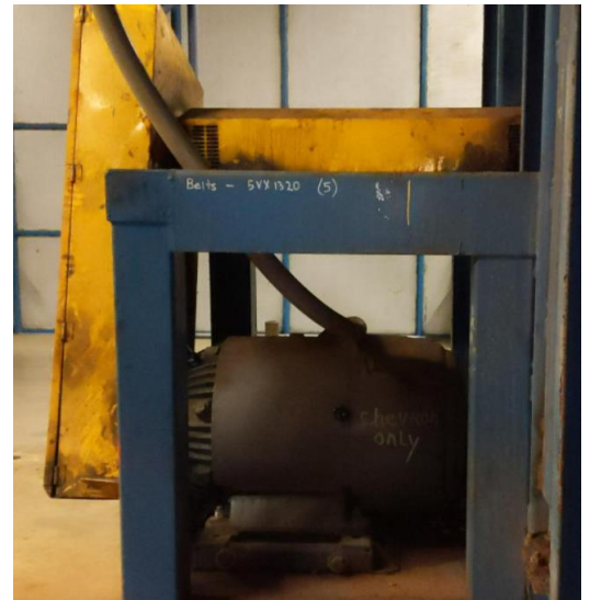
Exhaust fan at Ohio Assembly Plant
