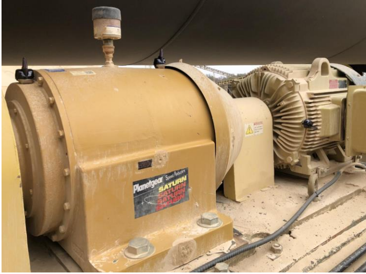
Above: Planetary Gearbox with two V3 Vibration Sensors
