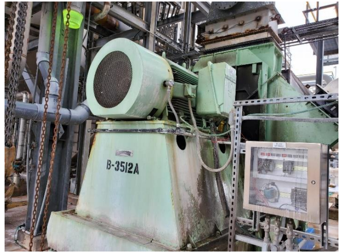
Figure 1: Dryer Blower in a Modifier Plant
